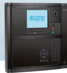
Fire alarm control panel
